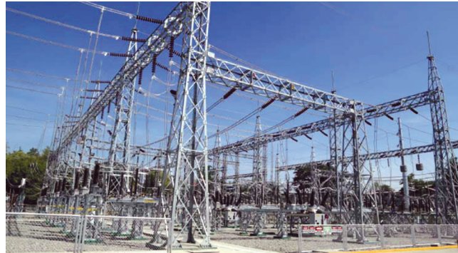
NGCP Transmission Towers. Source: NGCP
