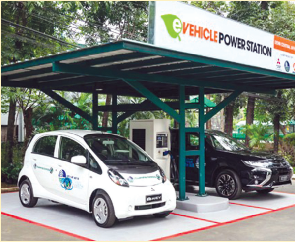
Electric charging station built in 2017 by Mitsubishi Motors Philippines and Meralco located inside the Department of Environment and Natural Resources Central Office.
