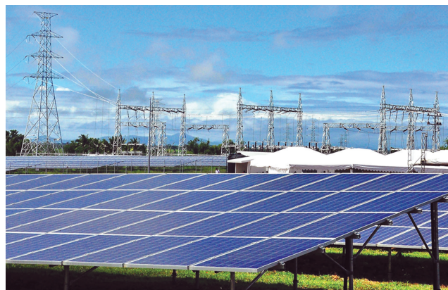
The 132.5 MW Cadiz Solar Power Plant is one of the largest in Southeast Asia located in Cadiz City, Negros Occidental. Source: Rappler.
